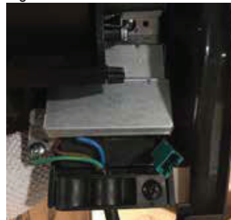
Figure 84: Terminal Cover Down.
